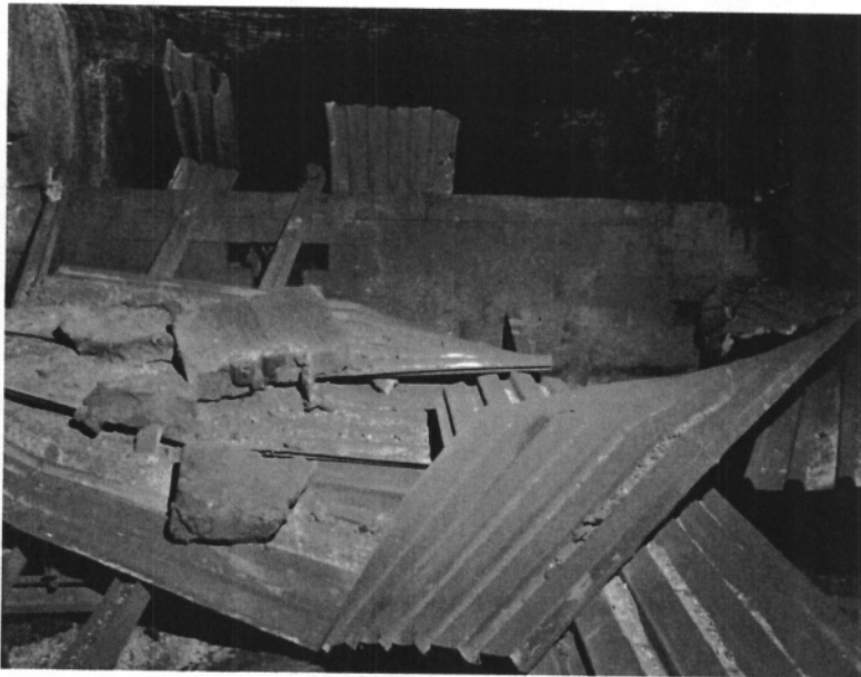
Ventilation overcast destroyed by the forces of the explosion.
