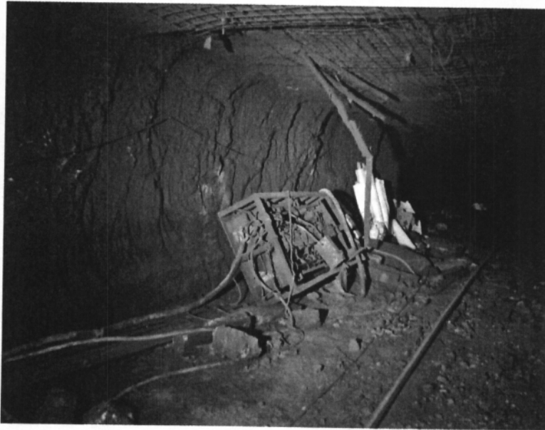
Damaged charging station located in the mains outby the sealed area.
