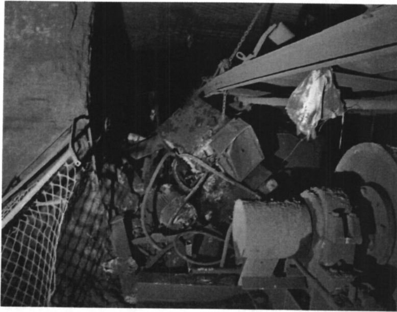
Damaged 2 nd Left belt drive. The drive was located at 58 block, approximately the location where the miners were forced to abandon their first rescue attempt.
