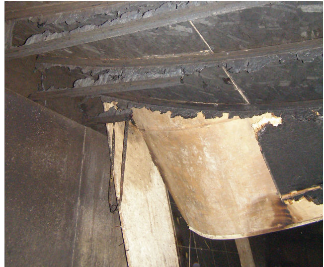
Figure 3. Fire-damaged I-joists where victim fell through floor. Note how the vertical web is almost completely consumed [NIOSH 2006a].
